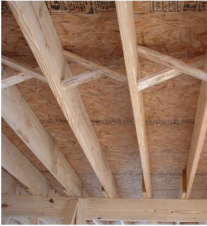
solid wood beams
