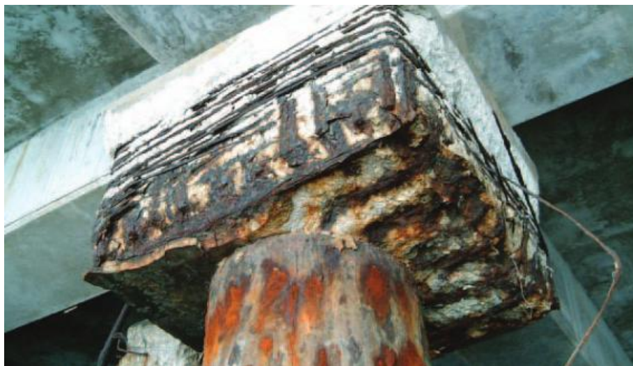
Fig. 1. Destruction of concrete and corrosion of reinforcement
